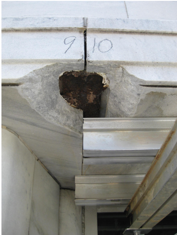
Failed Stone at eyebrow.
