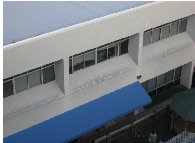
Distressed EIFS facade.
